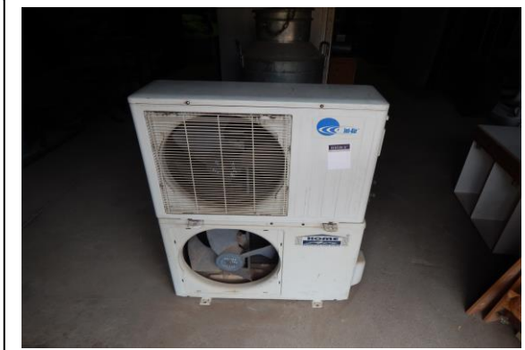
Aircon Outside Units
